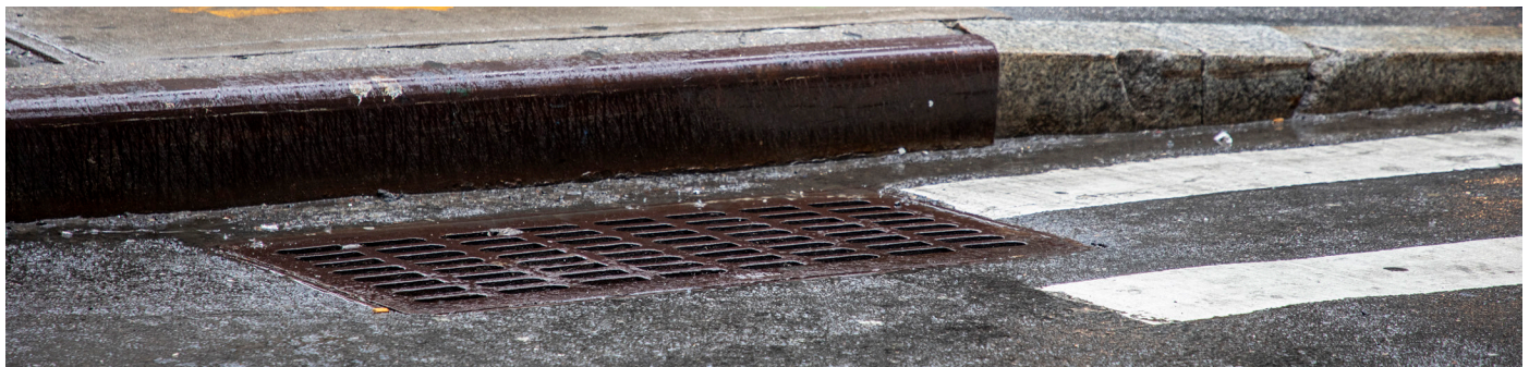
Figure 1: Typical catch basin (photo by Jean Schwarzwaldner)
